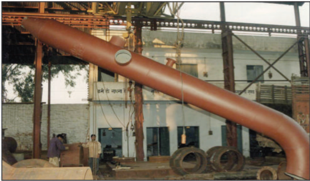
Turbine Integral Piping
